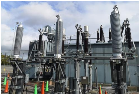
Ready to energize
